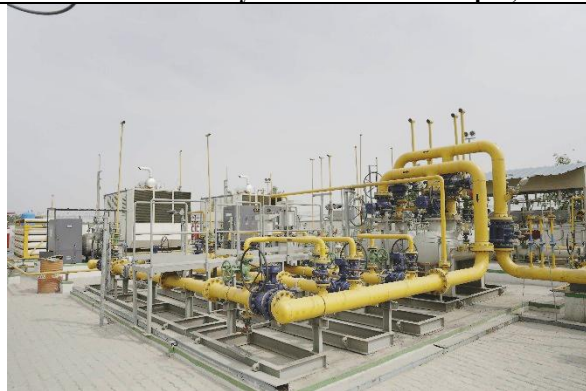
City Gate Station – Skid (pressure regulating and metering module)
