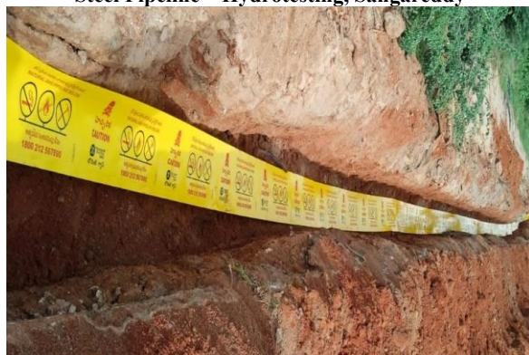
Steel Pipeline – safety mat, Sangareddy
