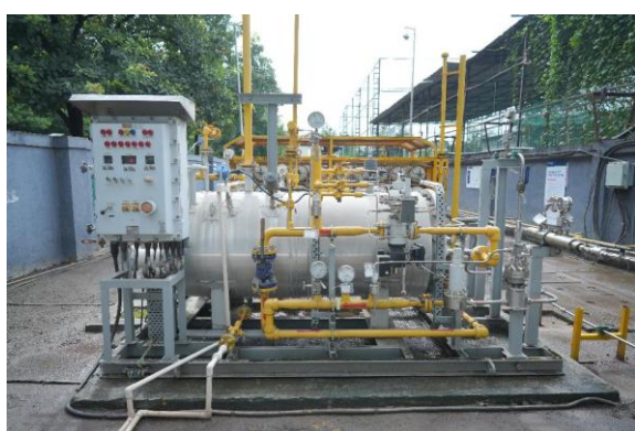
City Gate Station - Skid
