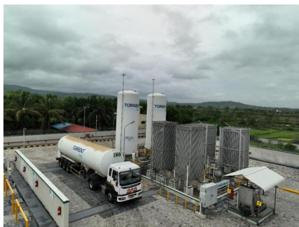
LCNG Station – Chennai
