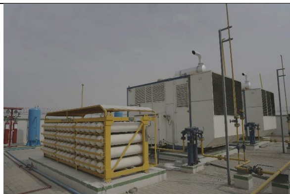
City Gate Station – Compressor (equipment that increases or maintains gas pressure to ensure reliable supply into the city distribution network)
