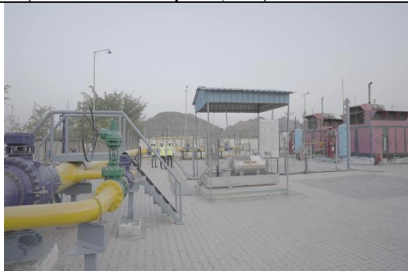
City Gas Station – Odourisation (safety system at the City Gate Station that adds smell to natural gas so that leaks can be detected)
