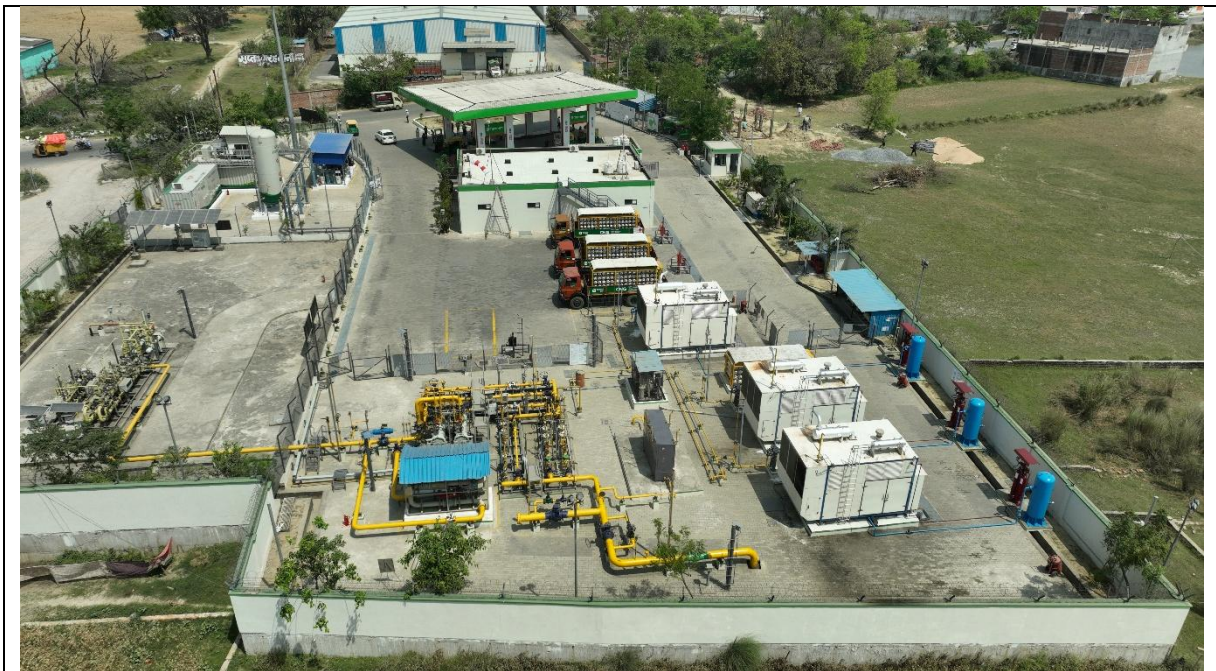
City Gate Station – Khanipur, Gorakhpur (Commissioned on April 30, 2021)
