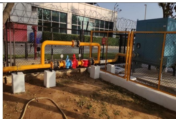
PNG Industrial Connection – Jaipur (Neemrana)
