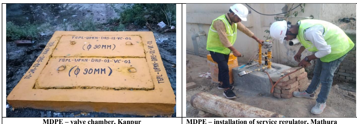
MDPE – valve chamber, Kanpur
